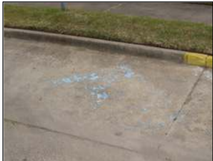
Image 2.5: Some handicapped parking is found in both on-street and off-street parking areas, but many markings have faded over time
